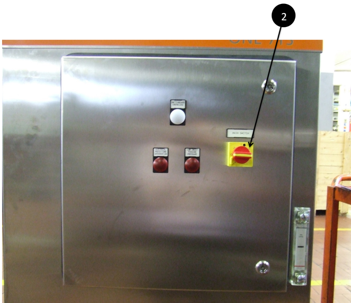
MAIN SWITCH FIG. 3.11
